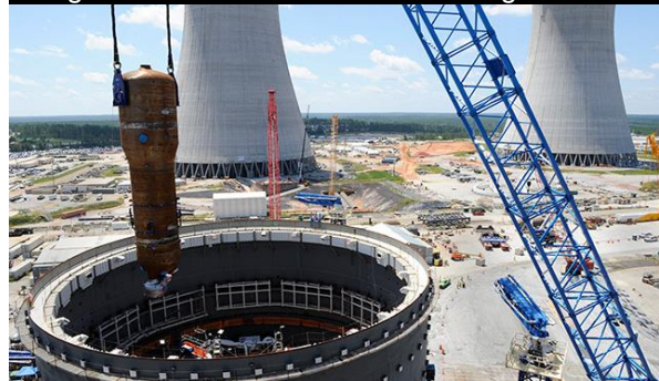
Vogtle Unit 3 Steam Generator – August 2017
